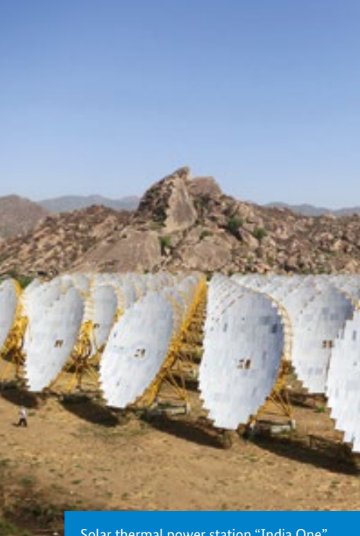
Solar thermal power station "India One", Rajasthan, India.
